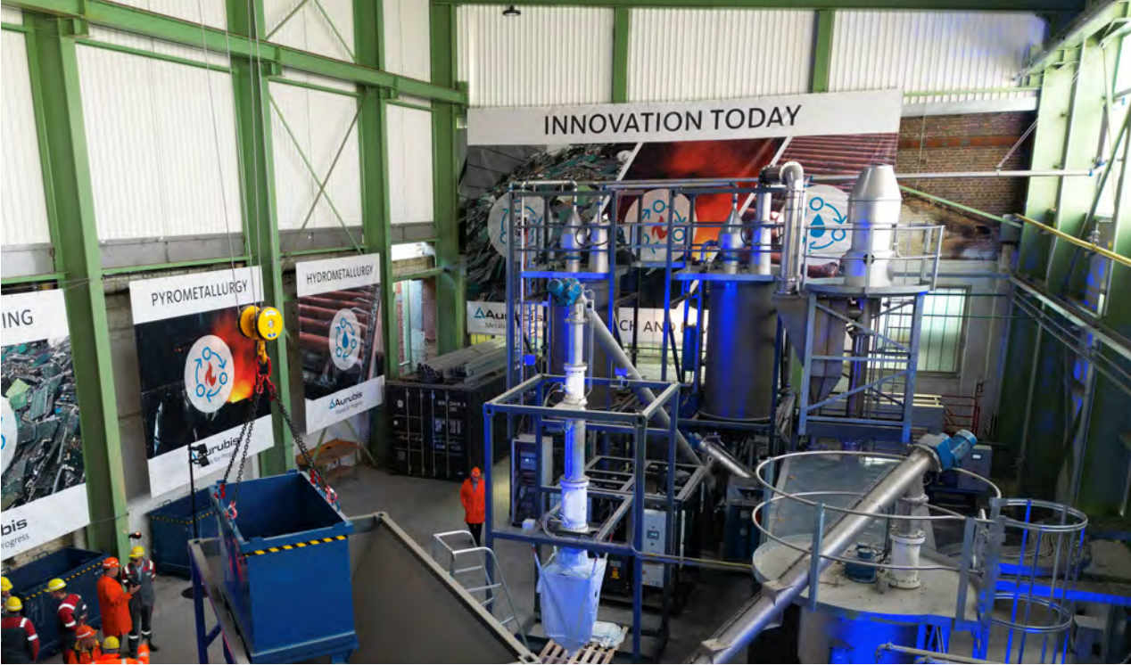
Pilot plant in Lünen: a pioneering role for new technologies.
